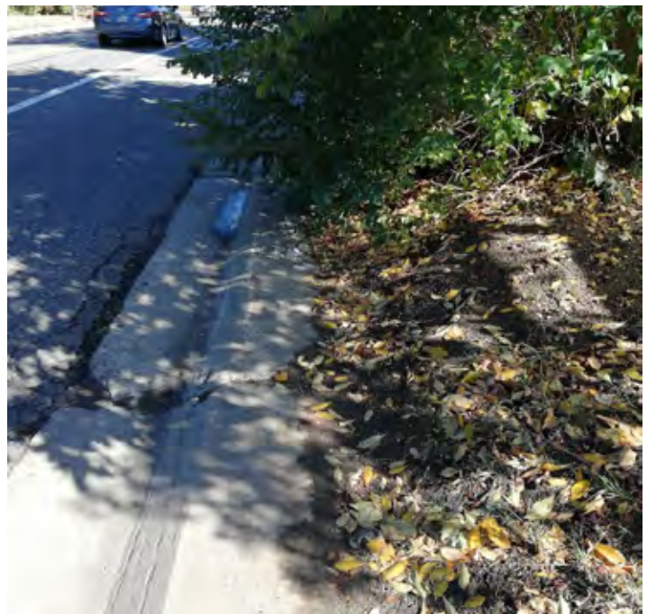
Exhibit 10. Obtrusion to Sidewalk on East 8th Avenue Near Busy Road
