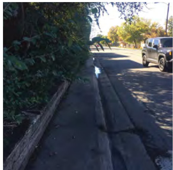
Exhibit 15: Sidewalk less than 3 feet roll-over curb
